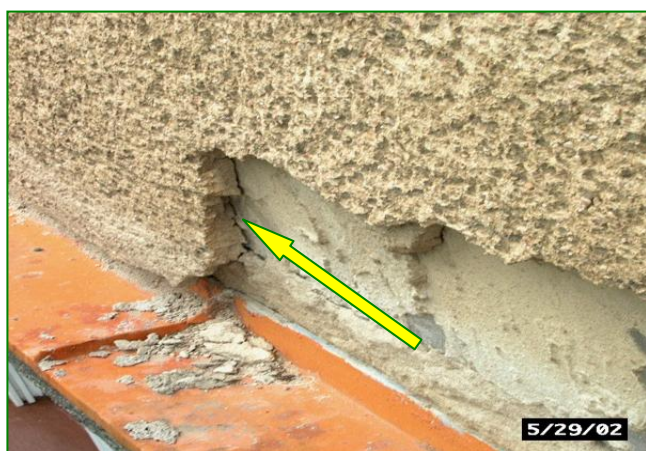
▲ Odpadnutá a oddelená omietka hrúbky 40 mm pri rímse Fallen off and separated rendering with thickness of 40 mm at the moulding
