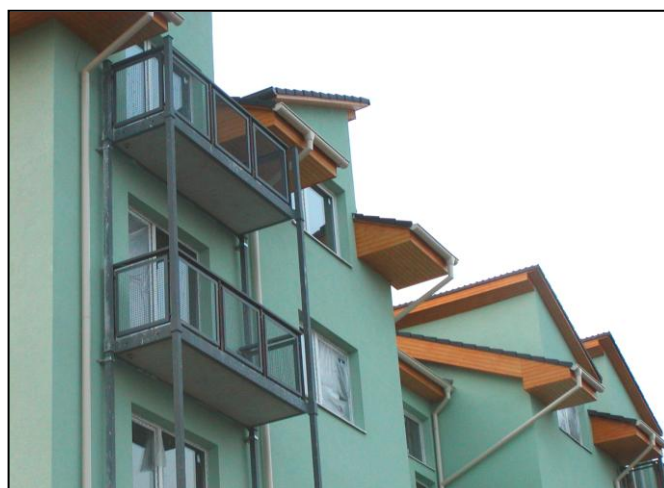
Detail ukončenia lodžií pri streche Detail of finishing of loggias at the roof
