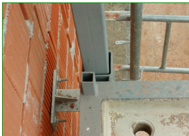
Detail spojenia stĺpikov a kotvenia zábradlia Detail of connection of columns and anchorage of railing
