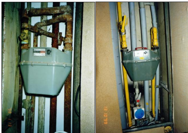
▲ Pôvodné inštaláčnne rozvody a po obnove Original installation distribution lines and after their upgrading
